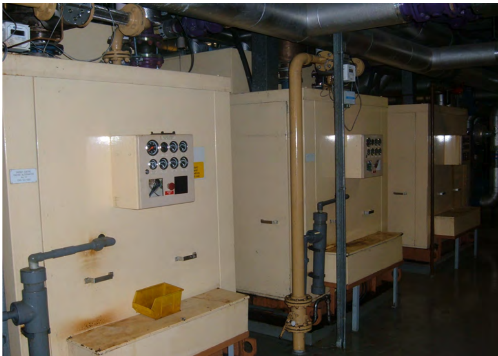
COMBINED HEAT AND POWER GAS ENGINE
